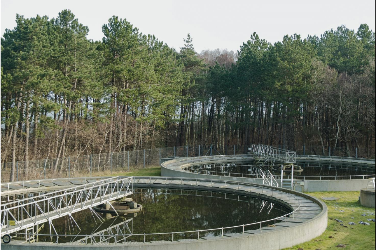
Figure 4.2: Hornbaek WWTP - one of three treatment plants along the coast
