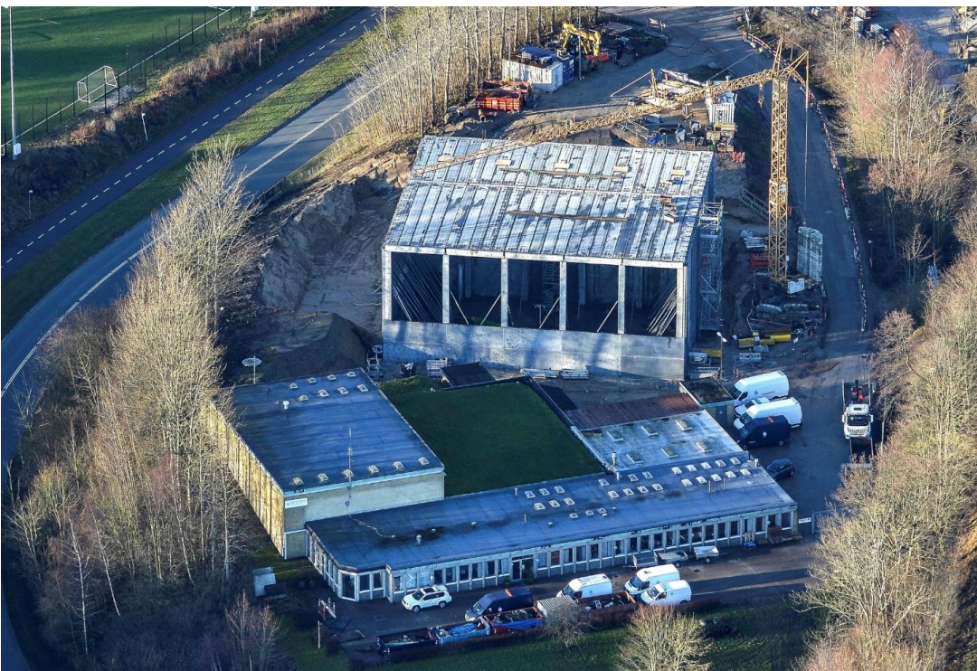
Figure 4.5: The new Snekkersten Waterworks under construction in winter 2019 (full operation since July 2020) behind the existing waterworks.
